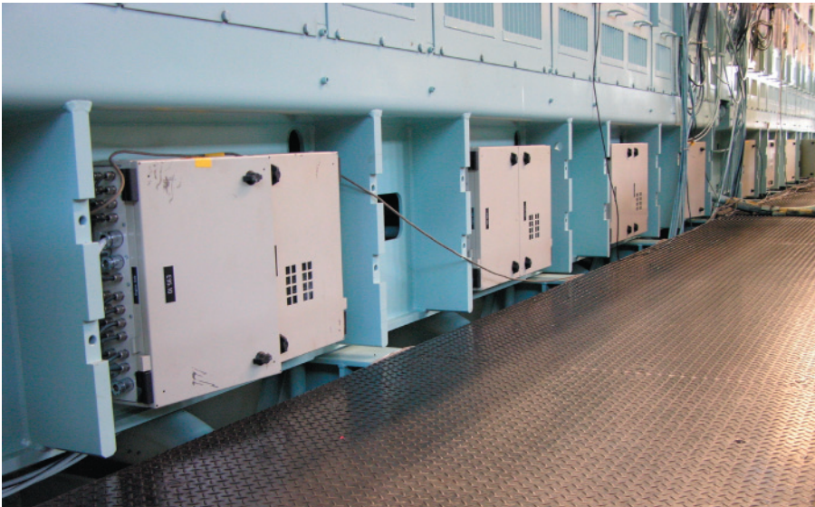
Fig. 16: Electronic control units beneath the front of the rail unit of a Sulzer RT-flex96C engine. [04#115]
