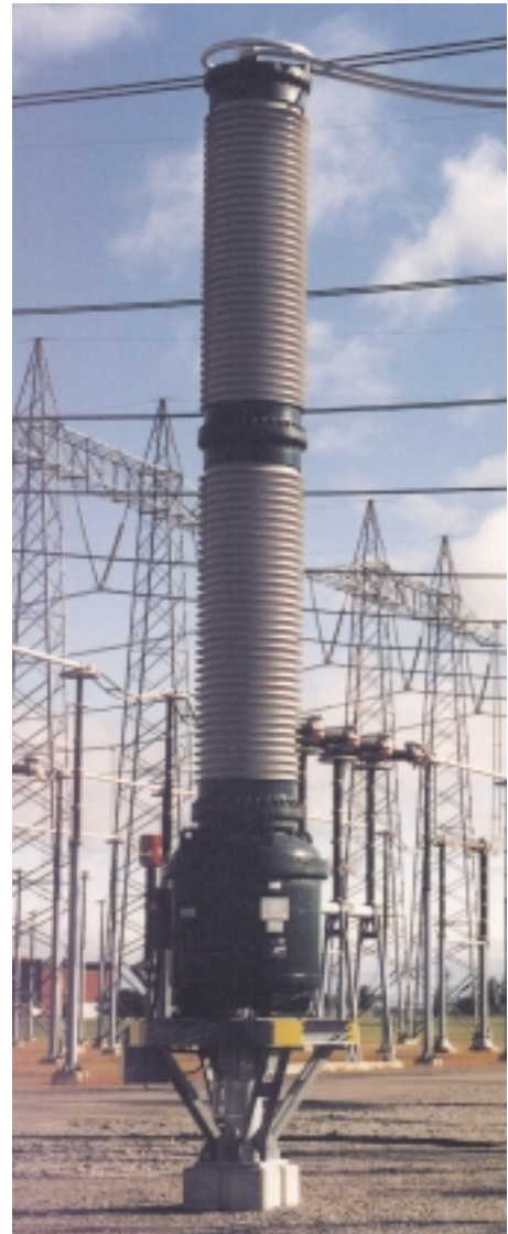
800 kV Voltage Transformer
