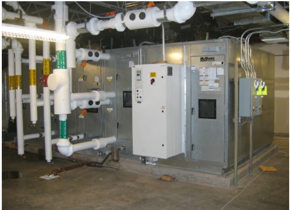
Four McQuay Vision indoor air handlers with energy recovery coils help to recover energy from the exhaust air stream and use it to pre-treat the supply air stream, helping to save on ventilation and energy costs.
